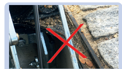
Fig. 10: INCORRECT: Sand on the seal and bearing surface
